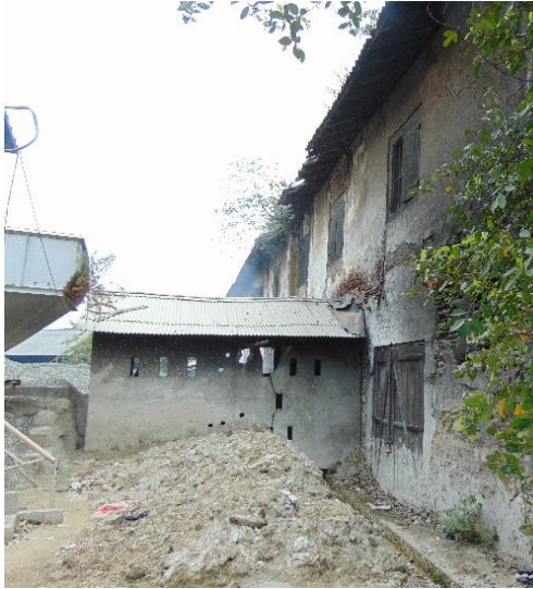
Left: small shop attachment to west side of grain warehouse (Photo by Pettman, 2015)
